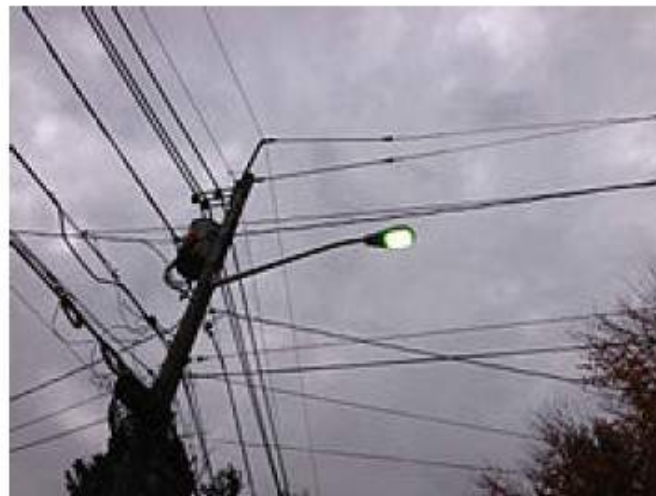
Mercury vapor street light
