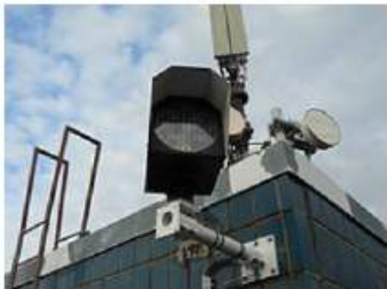
Laserlink point to point optical wireless network
